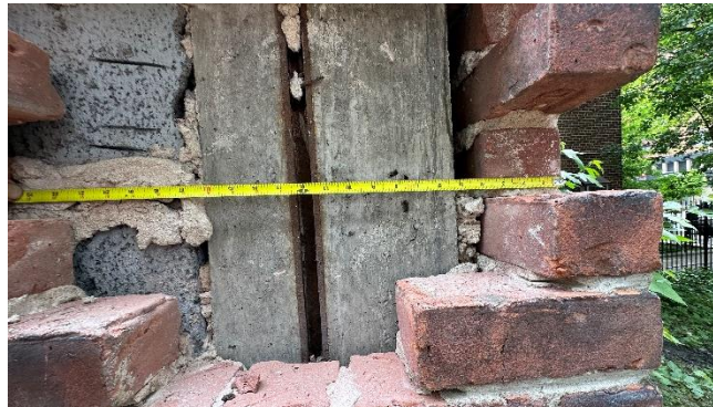
Corroded tie at Building 17
