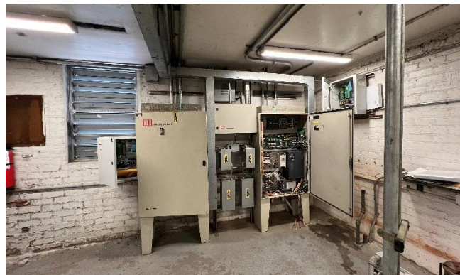
Building 5 Elevator Machine Room
