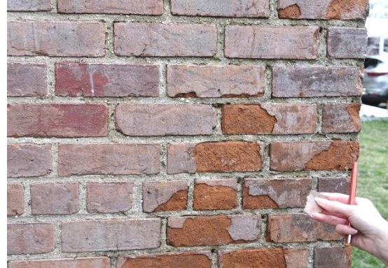
Spalling at Building 4
