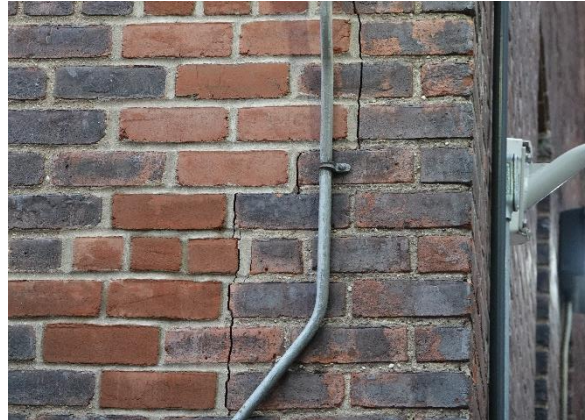
New crack at a previously repaired corner
