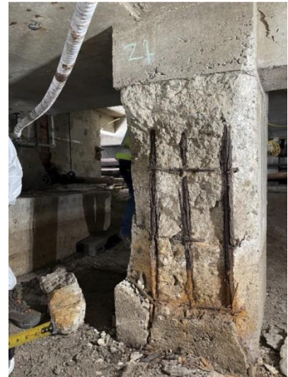
Deteriorated concrete at Building 9 crawlspace – photo by YAS
