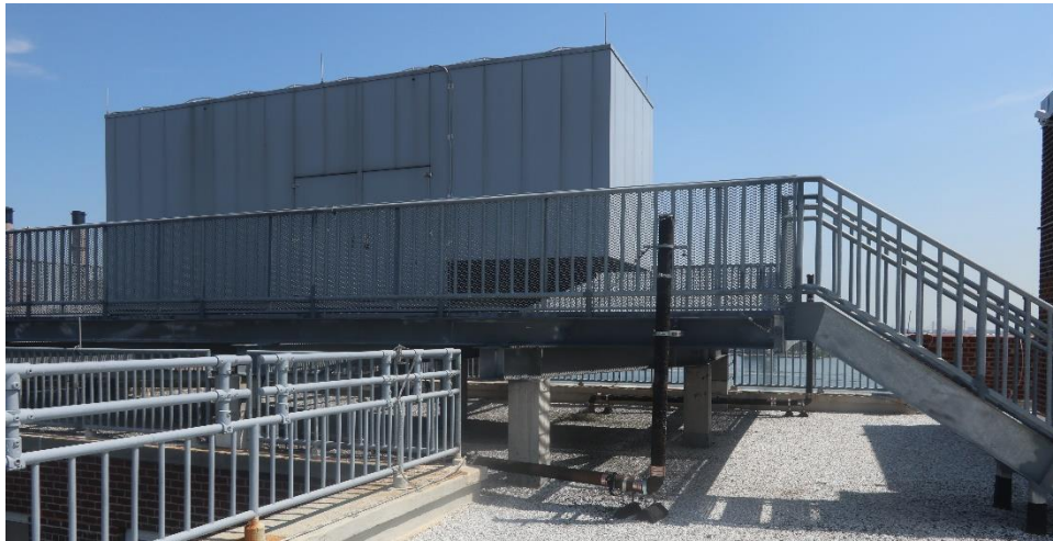
Roof generator at Building 14
