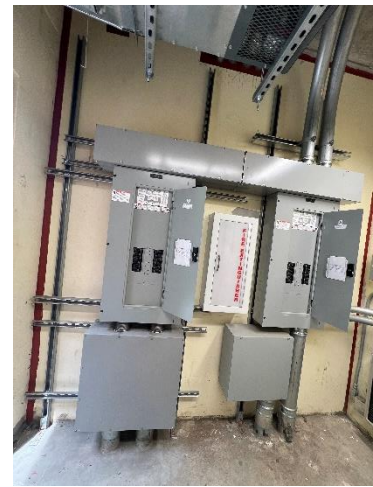
Electrical panel Room at Building 12
